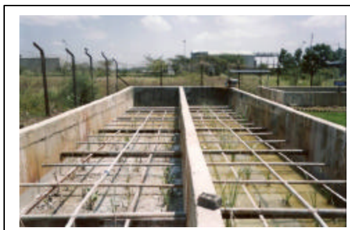
View of the Soil Scape Filter without plants. Wastewater is distributed on the top of Ecofert layer using grid of pipelines.
