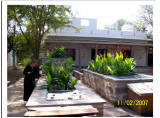
✚ A Soil Scape filtration unit at Narad Ka Baug, Amer, Jaipur.
